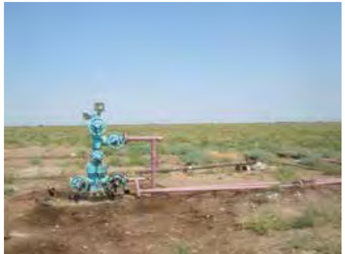
Typical Flowing Muradkhanli Oil Well
