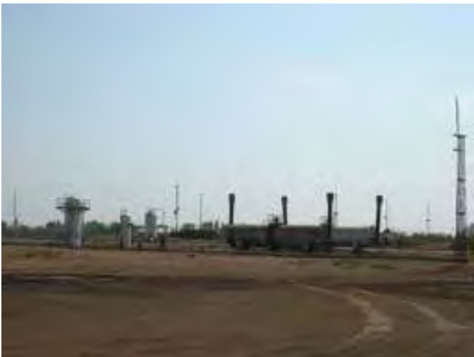
Heater Treaters and Other Equipment at Muradkhanli Central Facilities
